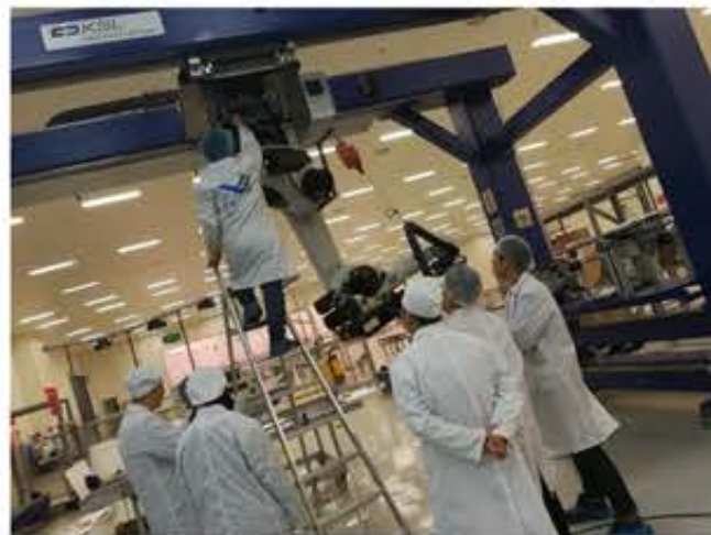
·SGG's technician team executed equipment installation at Shanghai Aircraft Manufacturing Co., Ltd.
